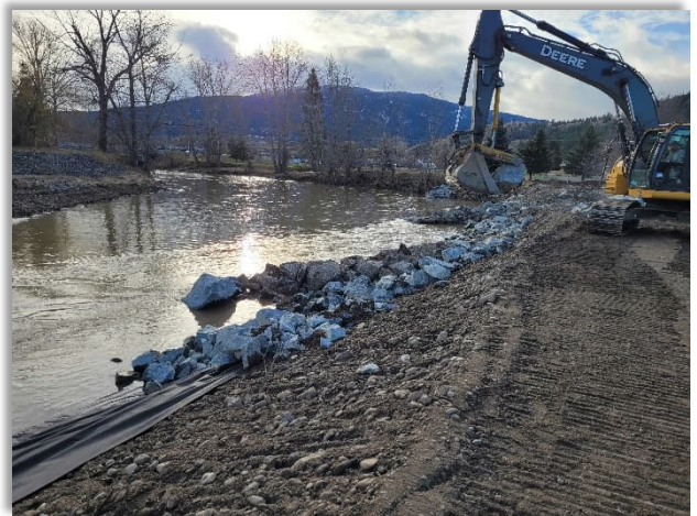
Temporary reconstruction of dike and bank protection at avulsion downstream of Main Street Bridge.
