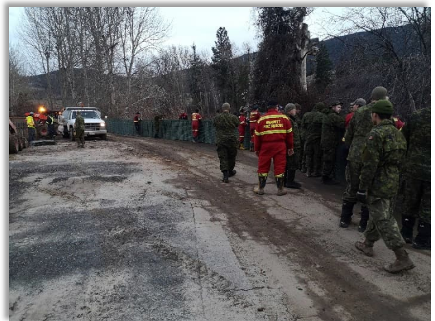
Merritt Fire Department and Canadian Armed Forces working together installing HESCO baskets.
