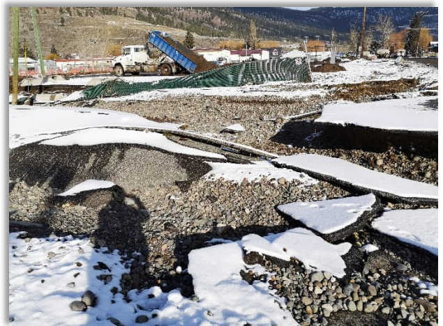
Road structure damage along Canford Avenue.
