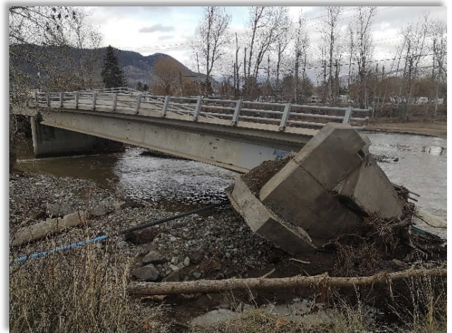
Collapsed span of Middlesborough Bridge.
